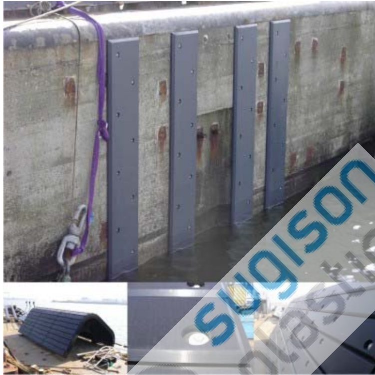
Fig. 4.d. Sliding Panels for Pier Protection
